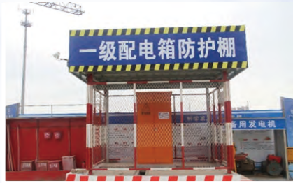
Power Distribution Board Shelter
