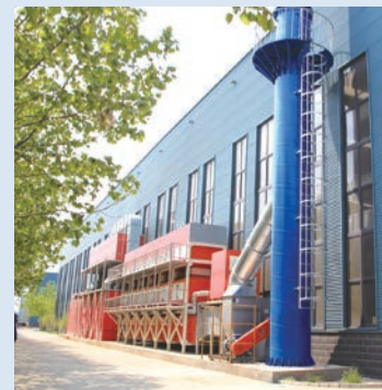
Paint spraying room
